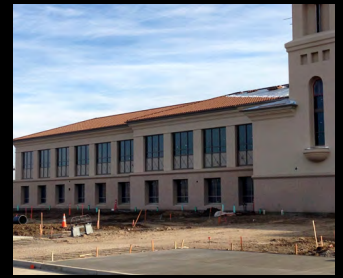
A must-open deadline kept Tarlton & Son workers hustling from March, 2013 until completed.
