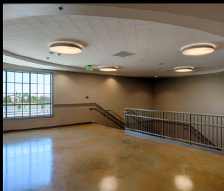
Curvilinear soffits add dynamic dimension and visual flow when traversing Mountain House High School hallways.
